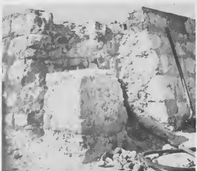
THE CORNERSTONE of Lago's original filter plant was set in place in 1925. Thirty-seven years later the sizable corner of coral was removed and saved for use in the demolition of the filter pool. The old walls give credit to the workmanship of the Aruban masons who constructed the reservoir in that the walls are as solid today as they were when built. E PROMER pidi di e Filter Plant original di Lago a worde poni na 1925. Trinta y siete anja despues e piedra grandi aki e work kibrá y warda ora e worde ducidi pa kibra e filter pool. E muryanan bieuw ta duna credito na e obra di man di mekai Arubano kende e traha e deposito aki pasaba e muryanan aparentemente ta mes firme ainda awe.
